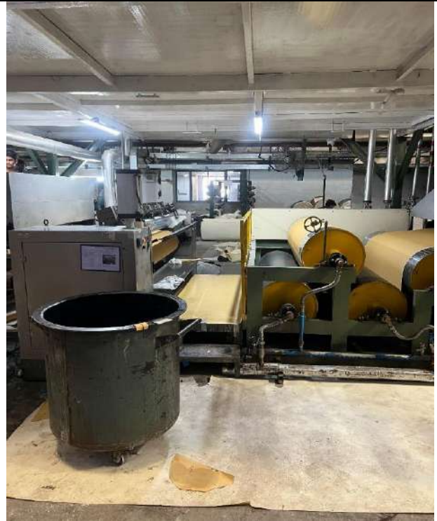
Machinery Name: Adhesive Head Location In Plant: Main Plant Use: Use water to cool down leather & paper temperatures
