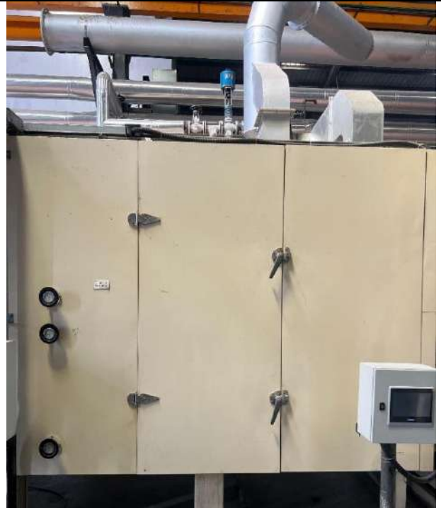
Machinery Name: 3Moven Location In Plant: Main Plant Capacity: To make PU or PVC slurry dry
